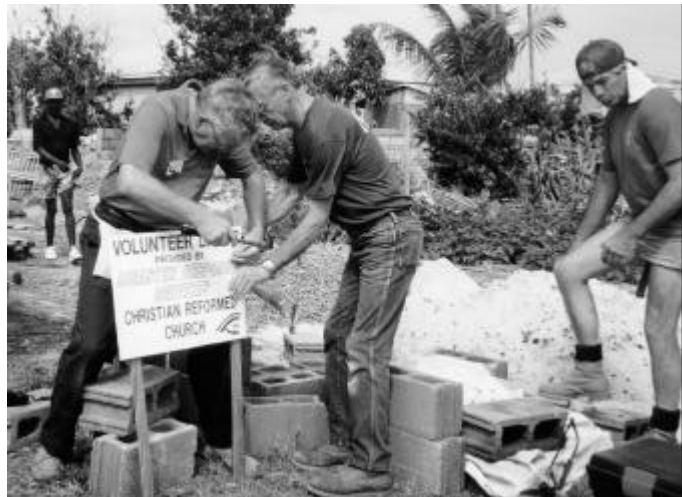
Volunteers from Christian Reformed World Relief Committee provide clean-up and rebuilding assistance in St. Croix following Hurricane Marilyn.
